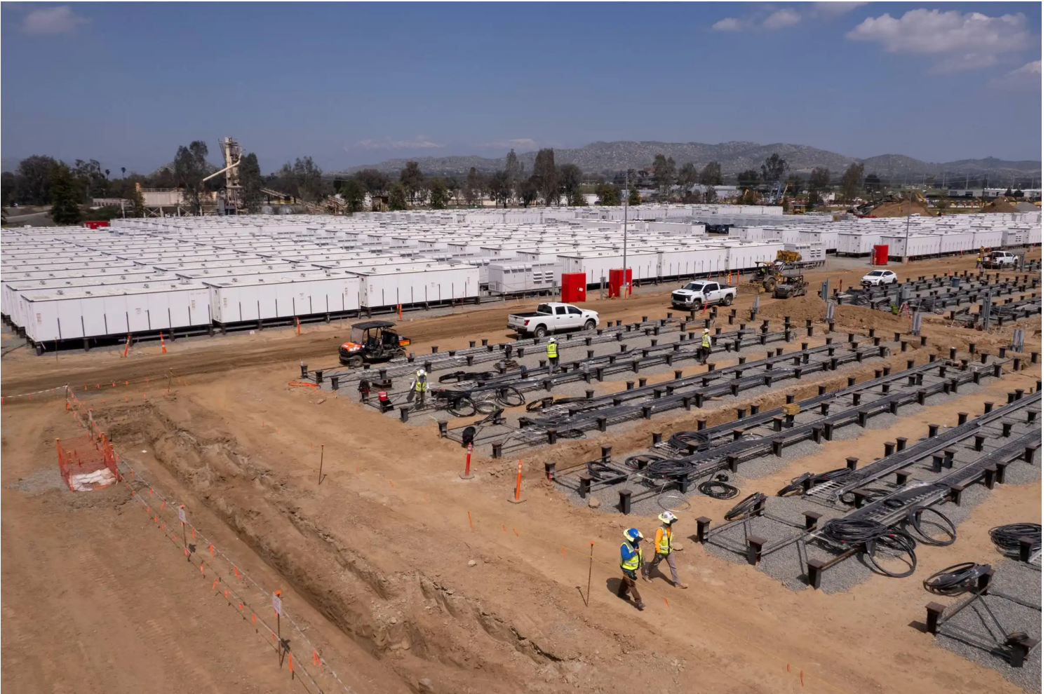
A battery storage facility under construction in Menifee, Calif., in March. The site, at 43 acres, is expected to be the largest in the state when completed. Mike Blake/Reuters
